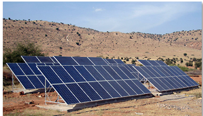
The solar pump system in Taroudant, Morocco is Africa's largest solar pump for irrigation.
